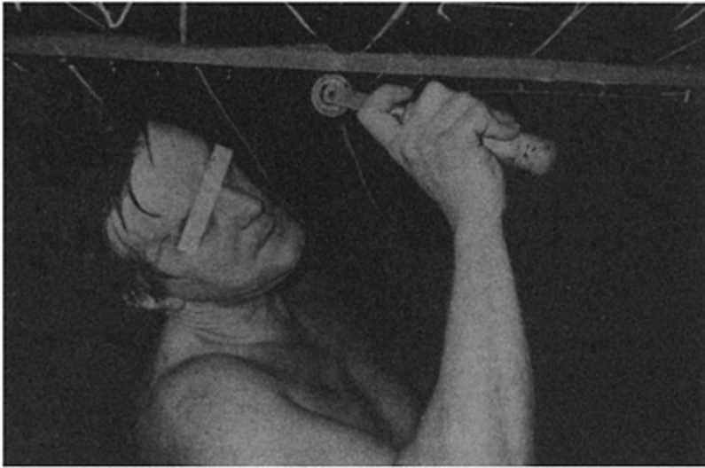
Figure 2: Application of rubber foil in an installation for exhaust fume desulphurization.
