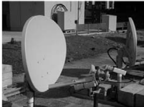
Fig 10.3 A VSAT (two-way) satellite antenna.
