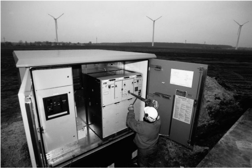
Figure 10.2 Transformer and Switchgear of 1.5 MW Wind Turbine, MV Switchgear on right, LV Switchgear on left (Reproduced by permission of NEG MICON; www.neg-micon.dk )
