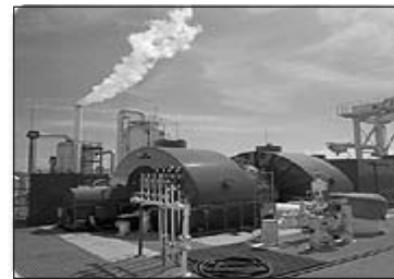
Fig. 2.32. Modern Geothermal Power Plant.
